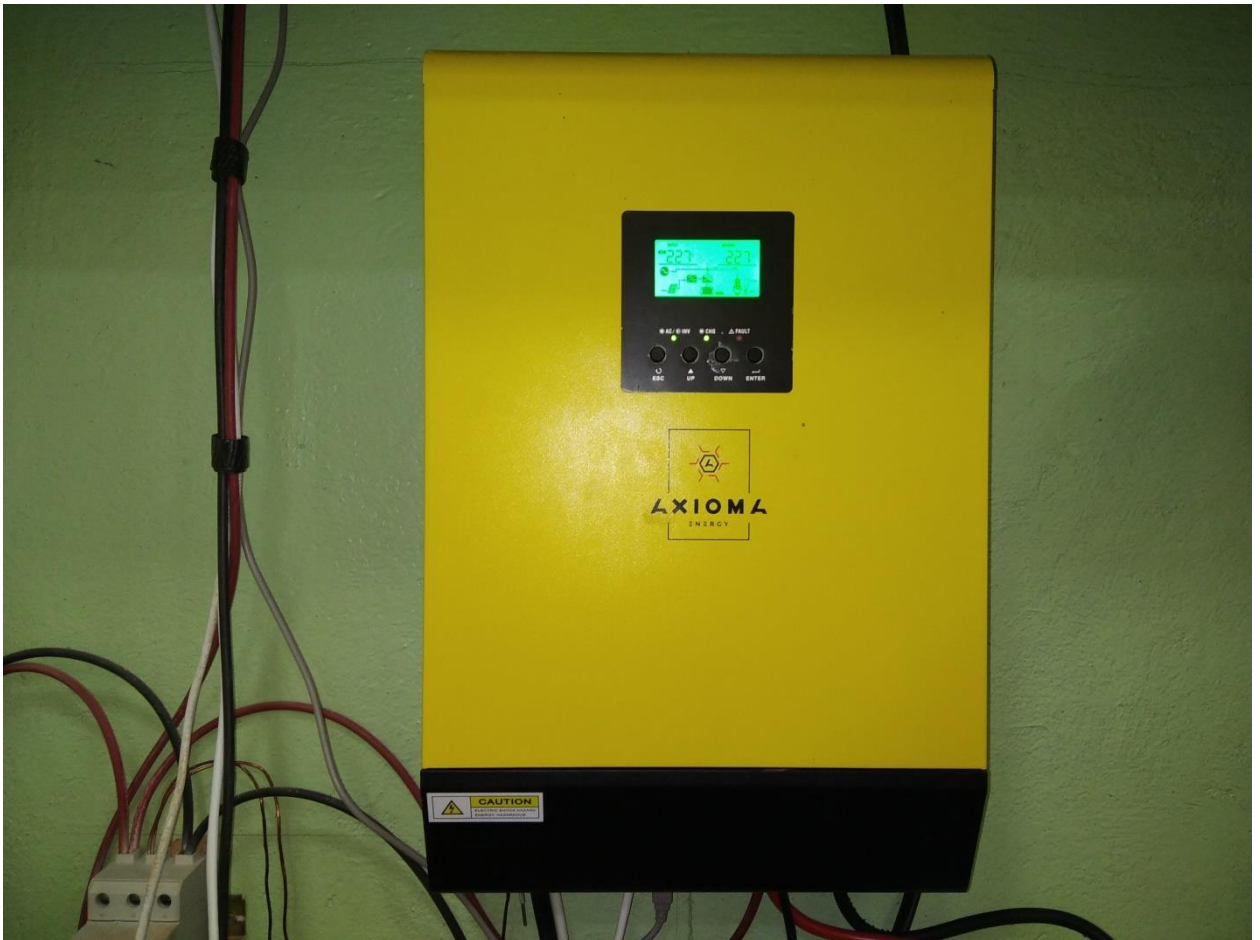
Fig. 2. Axioma inverter with connected block of photovoltaic panels, grid and rechargeable batteries.
